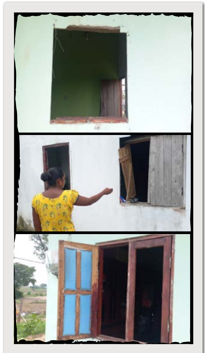
Elephant damaged homes
